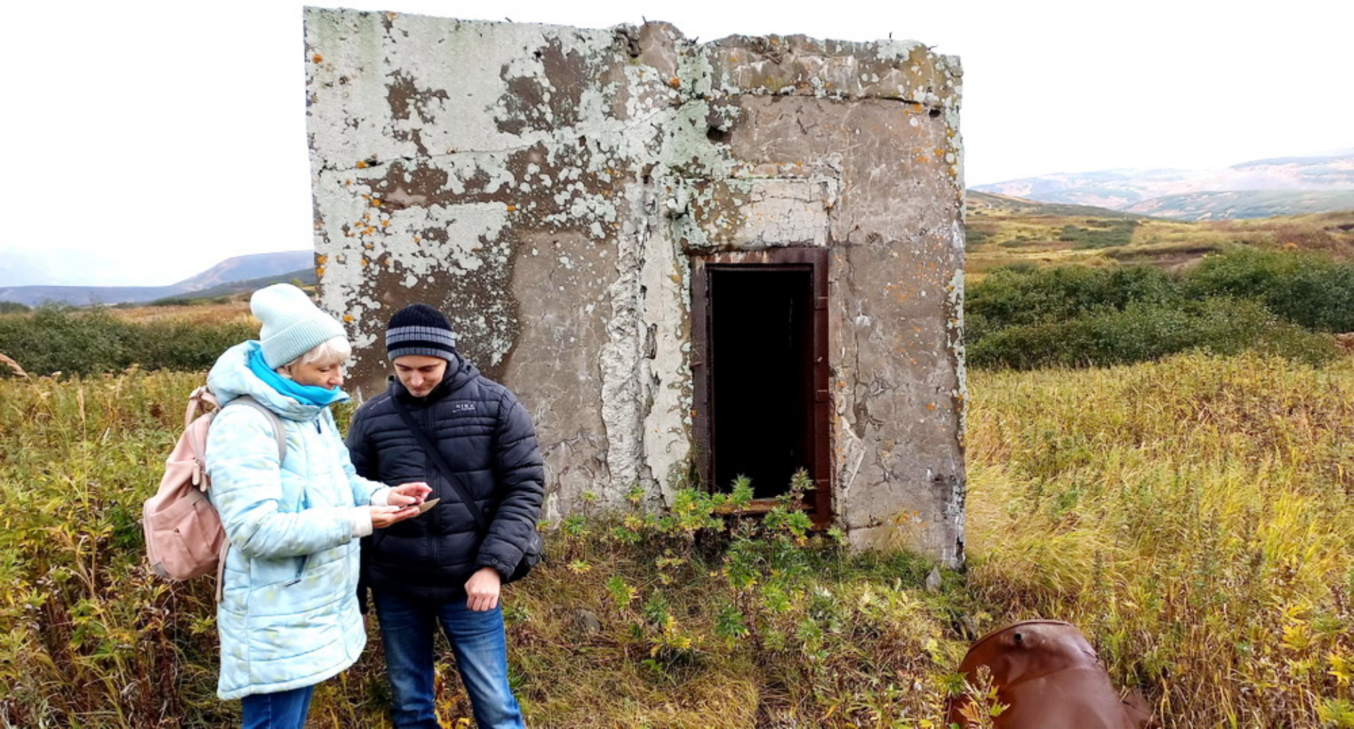
Severo-Kurilsk, September 2022. Concrete protective room in the state bank displaced on 1.5 km from the initial location
