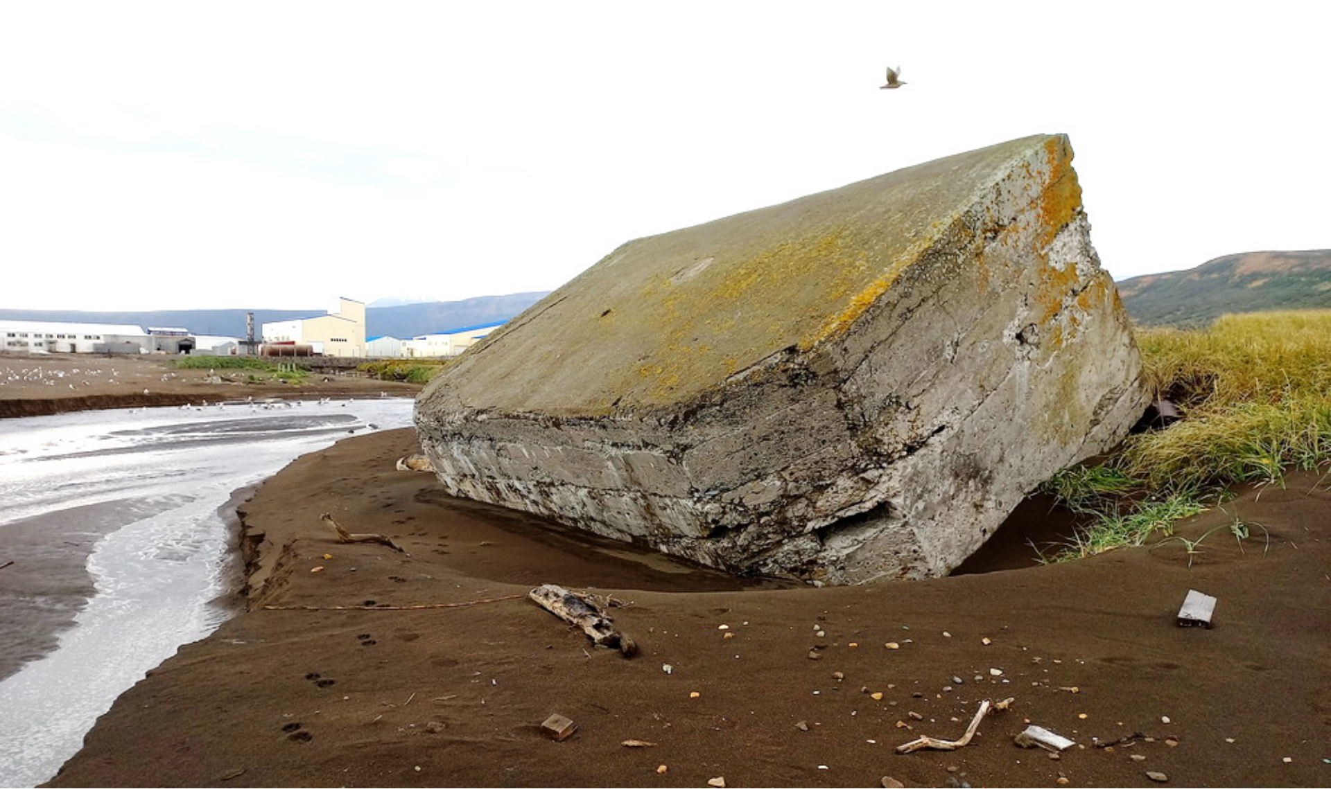
Severo-Kurilsk, September 2022. Concrete military defense unit overturned and displaced on several hundred meters upstream of a small river
